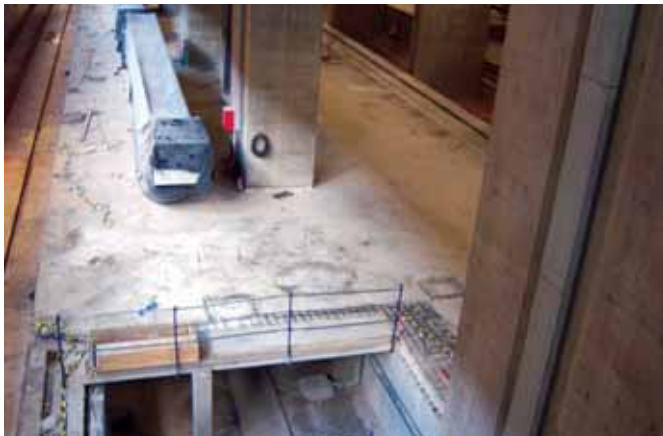
Madrid Barajas Terminal 4 - future regional rail platforms. Escalators have been delivered ut not yet installed. (Photo: November 2010)
